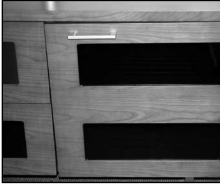
INCORRECT! Door is out of alignment with the rest of the unit.
